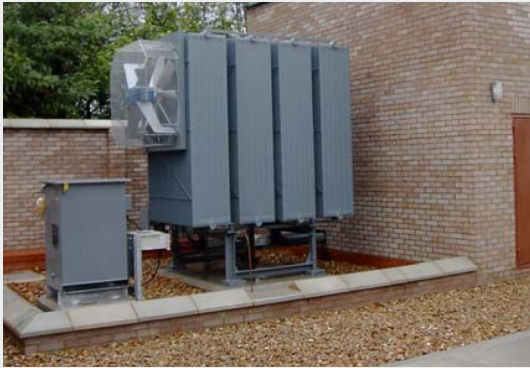
1 of 2 installed 12/24MVA 33/11kV Transformers
