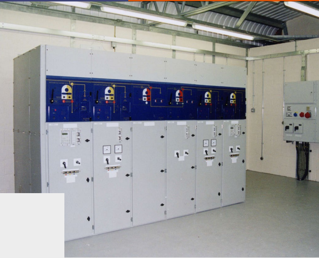
6 Panel 11kV Switchboard adopted by 24Severn
