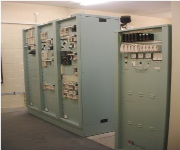
SPPOWERSYSTEMS SUBSTATION PROTECTION PANELS
