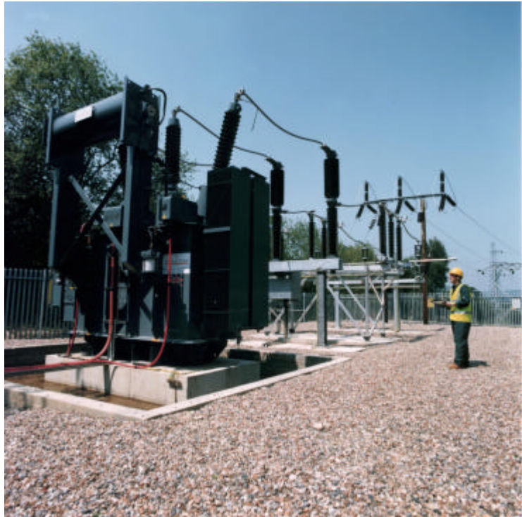
Stangate 132kV Substation compound
