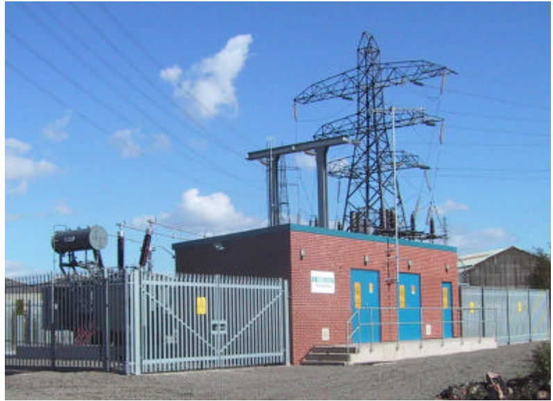
Simms Metals 132kV Substation
