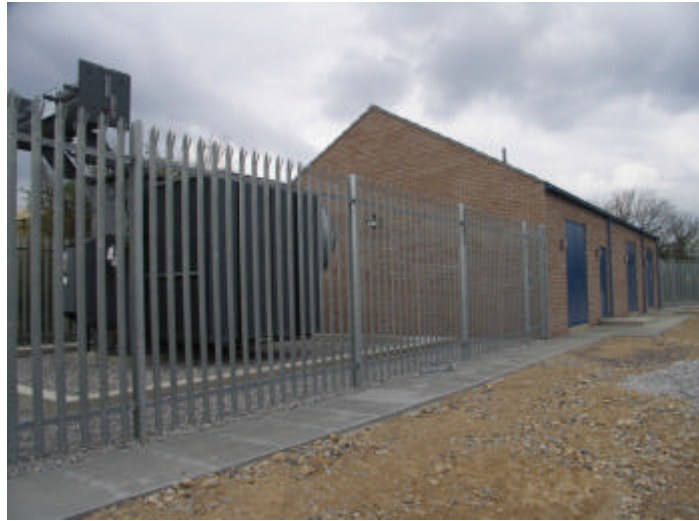
Corby Priors Hall 33/11kV primary substation
