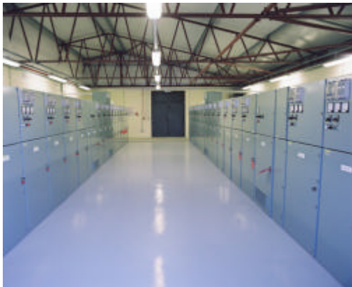
34 panel 11kV generator switchboard
