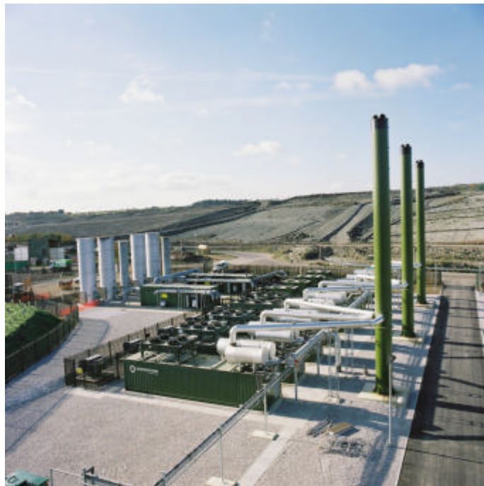
Brogborough Generation compound
