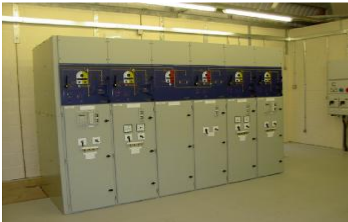
6 PANEL 11KV SWITCHBOARD ADOPTED BY 24SEVEN
