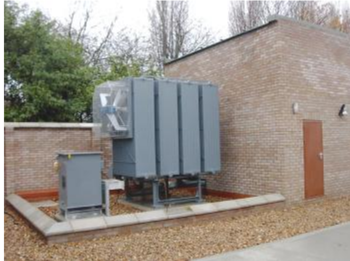
1 OF 2 INSTALLED 12/24MVA 33/11KV TRANSFORMERS
